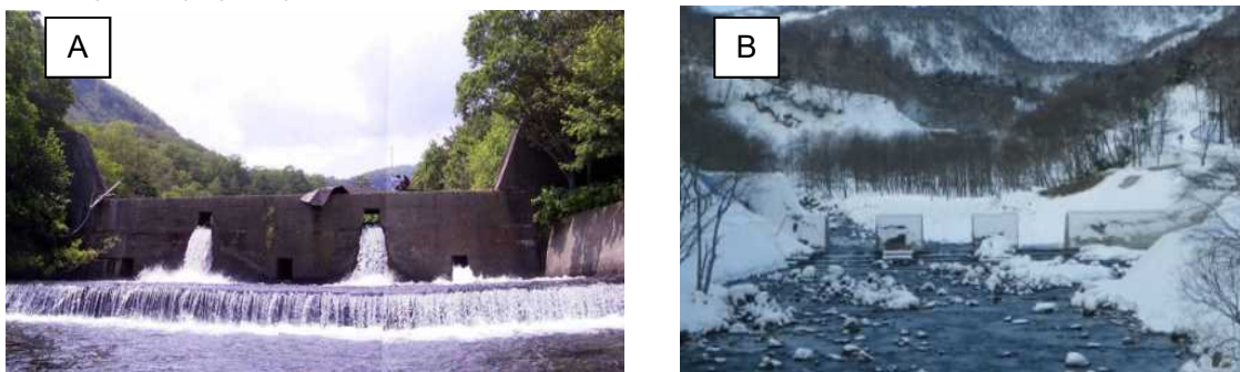
Fig. 10 Check dam before and after modification by making slits A: Before modification B: After modification
